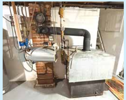
Original wood-fired unit on the right, with the electrical unit on the left.
